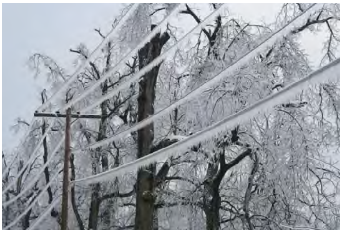
Figure 3-22 Ice Covered Power Lines
