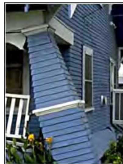
Figure 3-6 Earthquake Damaged Porch
